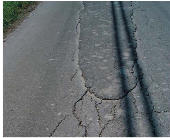
Longitudinal cracking and rutting, from localized base failure.
